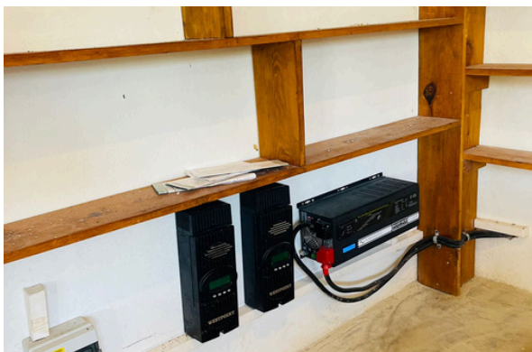
Solar inverters in the library/computer room will power new laptops!
