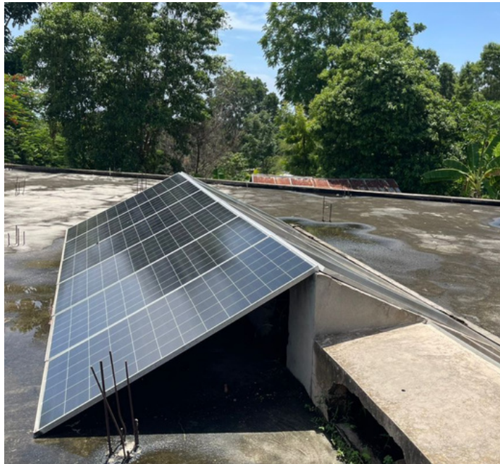
Solar panel on the roof of the BRHC
